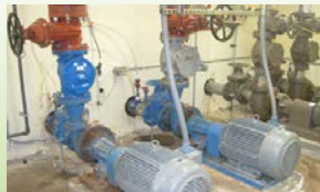
Booster Stations and Other Pumps
