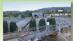
Wastewater Treatment Plant
