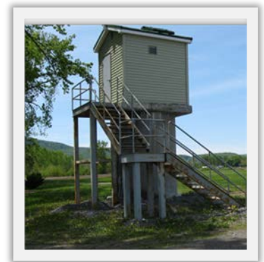
Wellhead above 100-year flood
