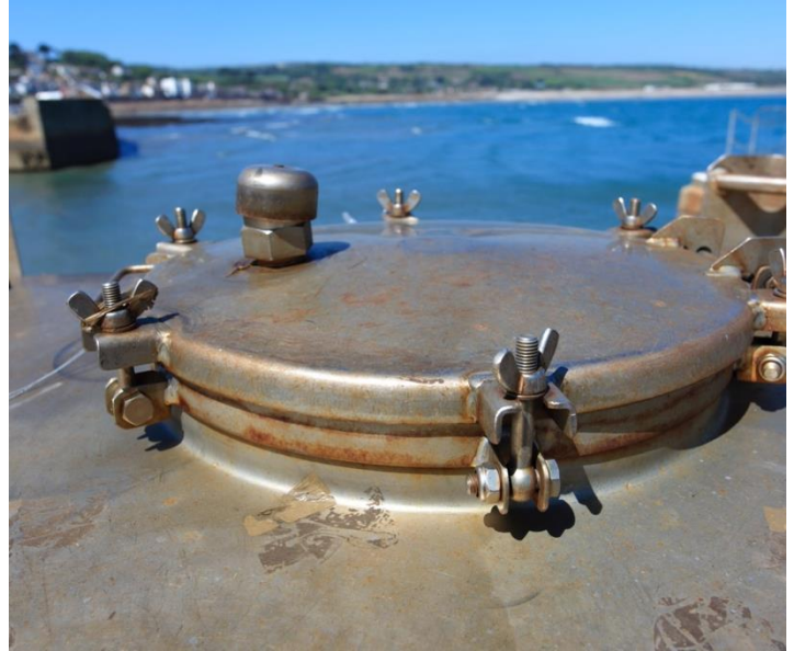
Example of a stainless-steel fuel tank with closure device secured in the closed position so that emissions are controlled.
