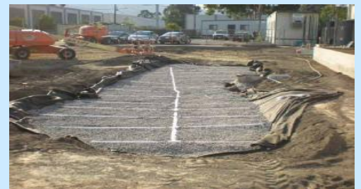
This underdrain pipe system will help to drain the bioretention area above it.
