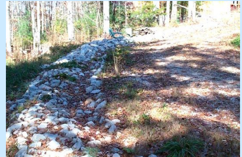
This diversion berm is constructed across a steep slope (max. 25% slope) to slow stormwater.
