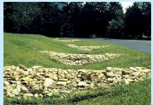
The rock check dams placed along this grassy swale help slow stormwater and prevent erosion in the swale (max. 6% slope).
