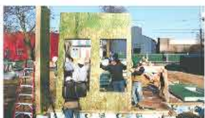
CONSERVING ENERGY New homes built on the Near West Side use insulated panels.
