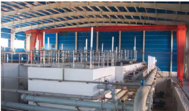
Figure 2 Beijing MBR facility (Photo credit: Courtesy of GE Water and Process Technologies)
