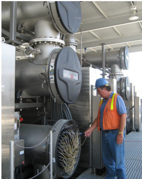
Figure 3 GWRS ultraviolet reactor system (Photo Credit: Gina DePinto)
