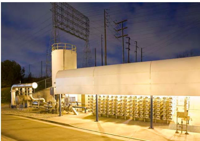
Figure 2 Reverse osmosis treatment at the ECLWRF
