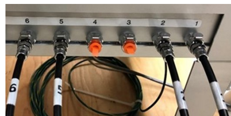
Disconnected and capped lines at the pump box
