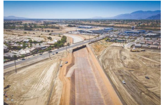
North Indio Regional Flood Control Project Photo Credit: Coachella Valley Water District
