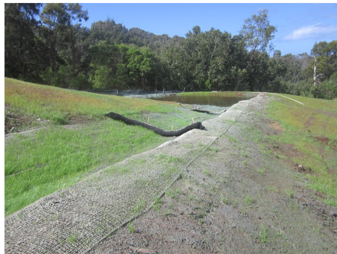
Compost filter socks installed in a vegetated channel leading to a sediment basin.
