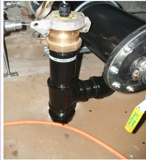
Figure 6.2. Another notable variation for the design of a category 3 system involves a liquid-detecting cable run within the length of the piping interstice.
