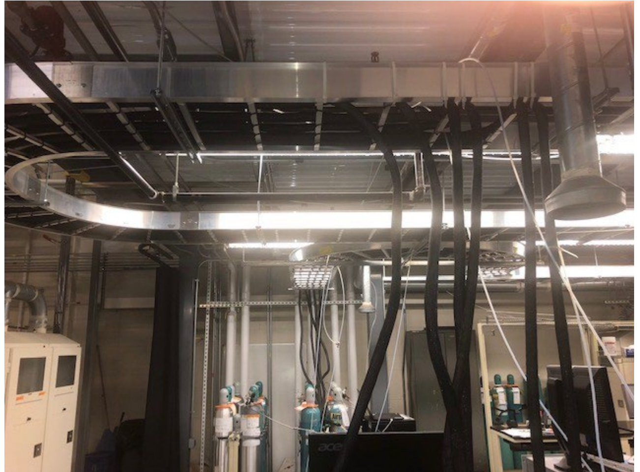
Heated line test rack
