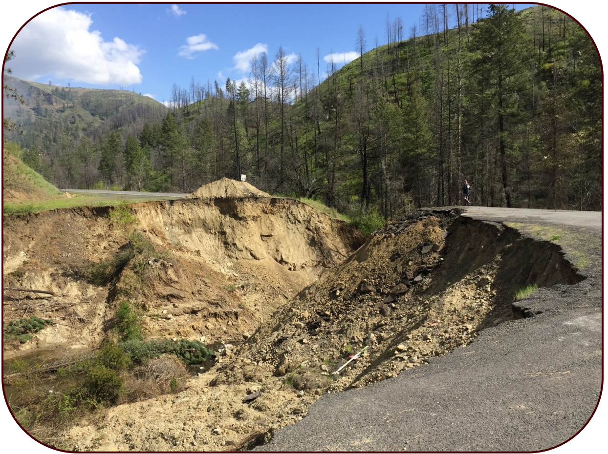
Tom Taha Road Damage from flooding in April 2019 from major disaster declaration for Idaho (HQ-19-057) (Copyright: Nez Perce Tribe Water Resources Division)
