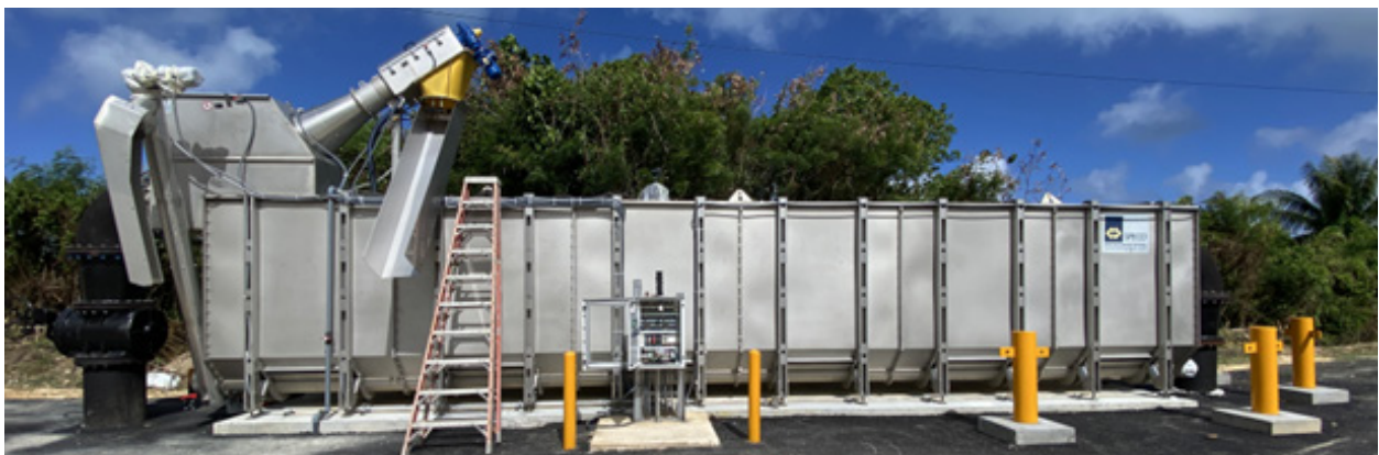
Primary screen at the Sadog Tasi Wastewater Treatment Plant
