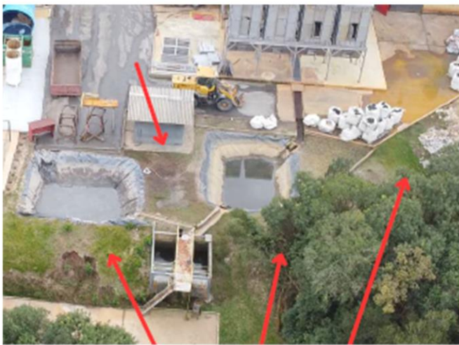
WWTP with signs of overflow - lack of containment of the lagoon
